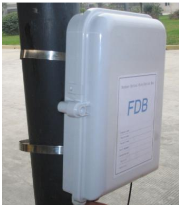
FTTH-005 fiber termination box on the pole
