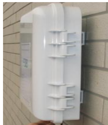
FTTH-005 fiber termination box on the wall
